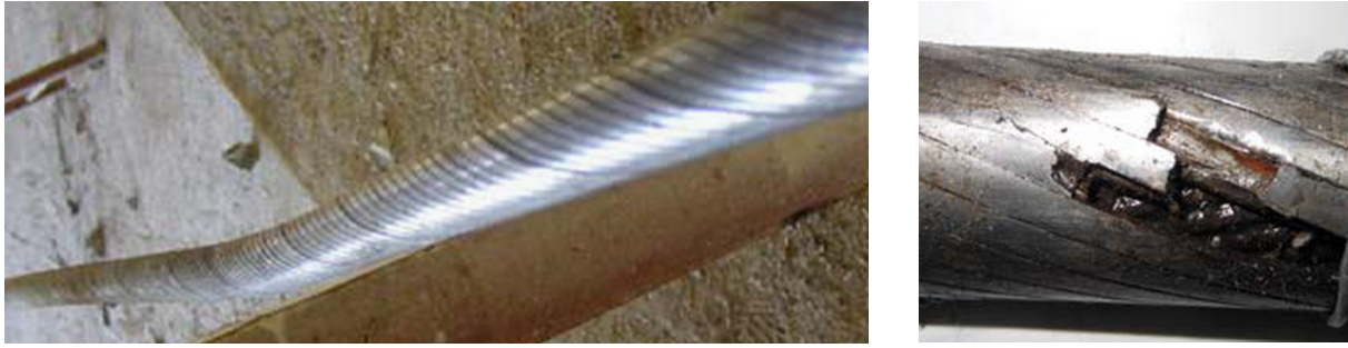
Fig. 1. The view of the damaged rope, a) the release of the Z wires from the surface layer, b) the nest of the ruptures of the Z wires from the surface layer
