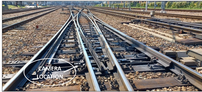
Figure 23. Location of the camera setup for observing vertical movements of the stock rail in a double slip turnout during the passage of passenger rolling stock
