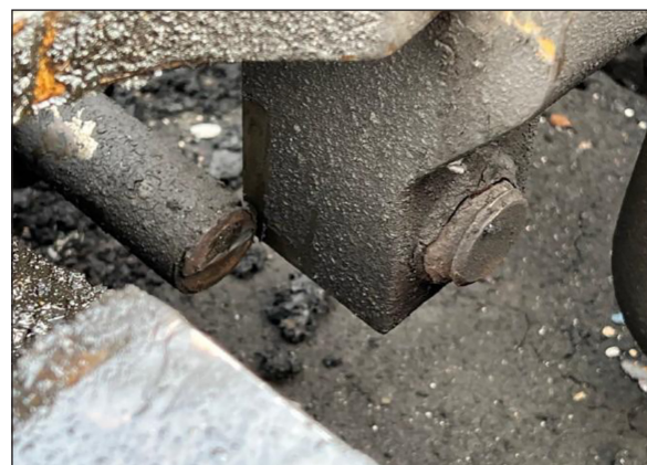
Figure 10. An example of a broken coupling rod at the fixed bracket location
