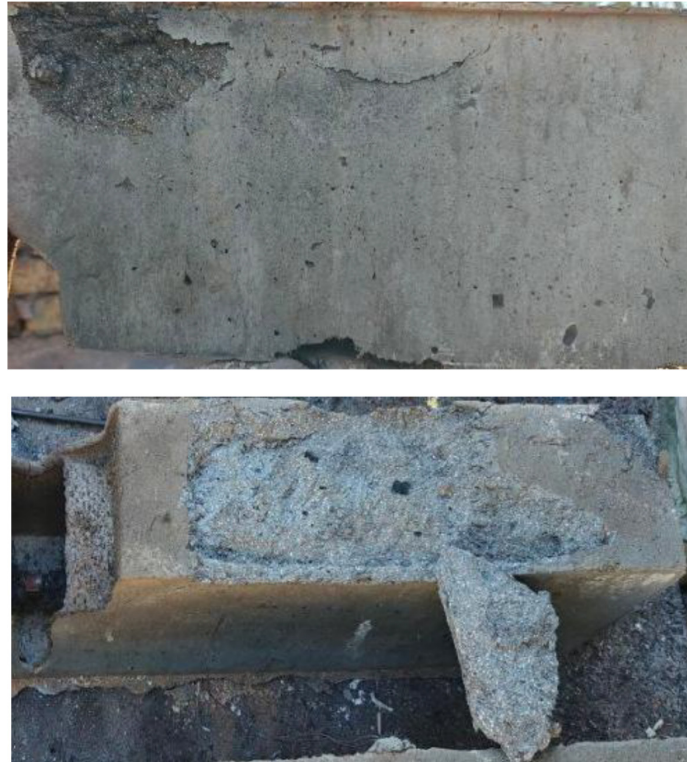
Figure 10. Spalling after exposing to 600 °C
