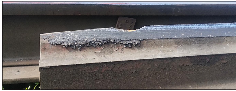
Figure 6. Example of breakouts on the switch rail
