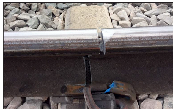
Figure 6. A broken rail caused by a tiny defect in the foot of the rail and repeated bending under traffic [11]
