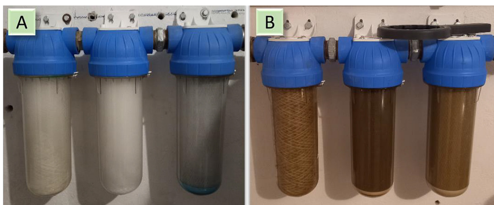
Figure 10. Whole-house filtration system consisting of 3 filters (filters from left to right: yarn, spun, carbon): A – clean filters immediately after installation, B – dirty filters requiring replacement
