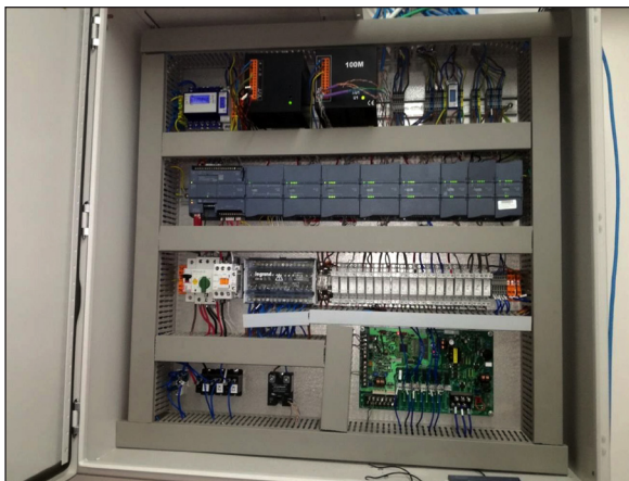
Fig. 18. Control cabinet [Photo: P. Obstawski]
