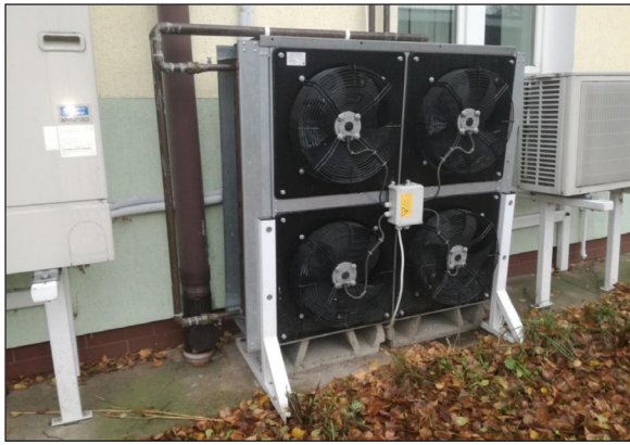
Fig. 16. Fan cooler installed outside the building [Photo: P. Obstawski]
