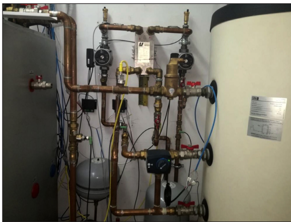
Fig. 17. Three-way mixing valve with plate heat exchanger [Photo: P. Obstawski]
