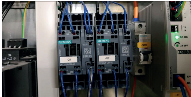
Fig. 6. Contactors supplying the respective conveyors
