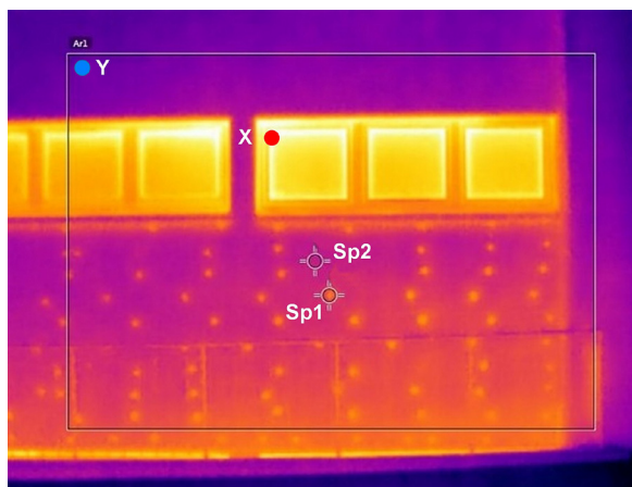
Fig. 2. Spot thermal bridges caused in fixing foamed polystyrene panels for facades
